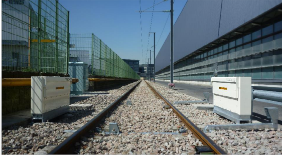
BEARING ACOUSTIC MONITOR
