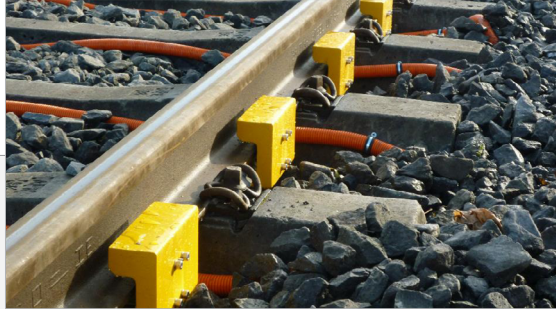
WHEEL CONDITION MONITOR
